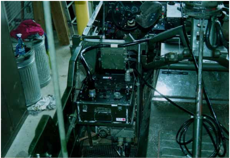
Figure 3-1-4: MGS Power Conditioner and TI Sight Power Conditioner
